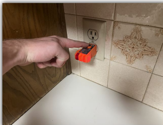
Missing GFCI protection in kitchen area
