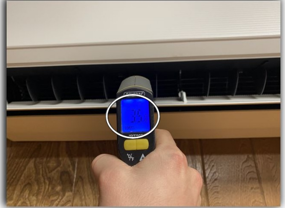
Supply air / differential
