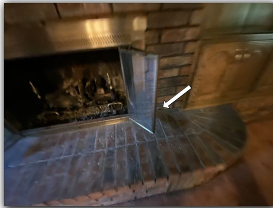
Gas working as should.
