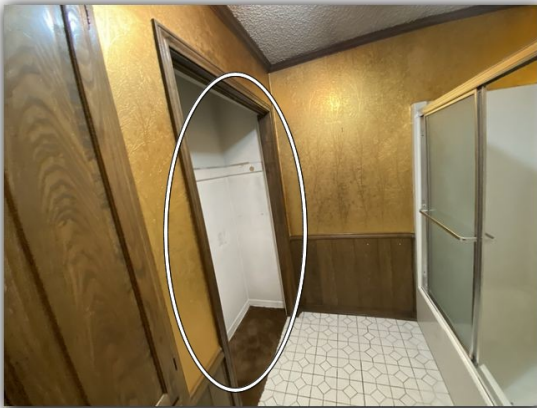
Hallway bathroom closet
