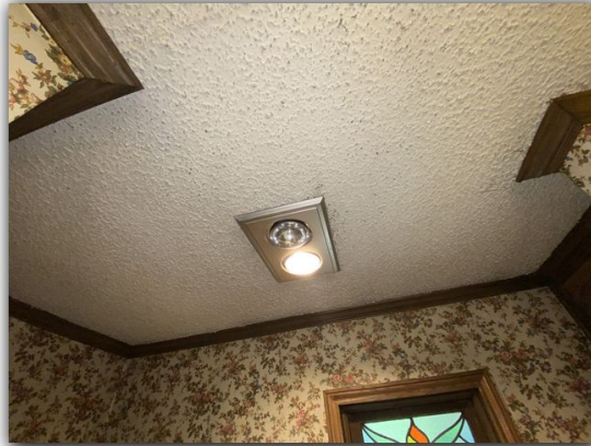
Bathroom heaters working as should.
