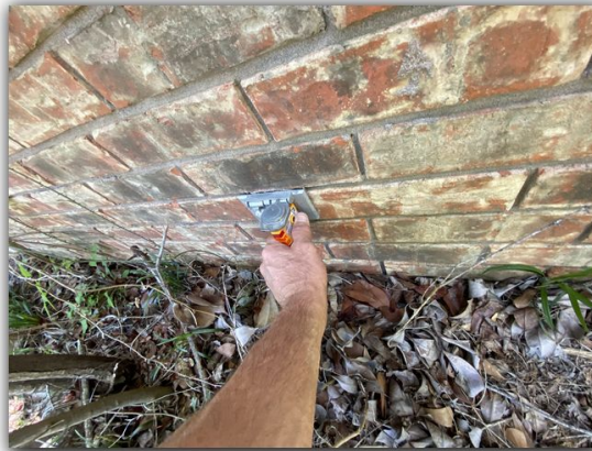
Missing GFCI protection on exterior of home
