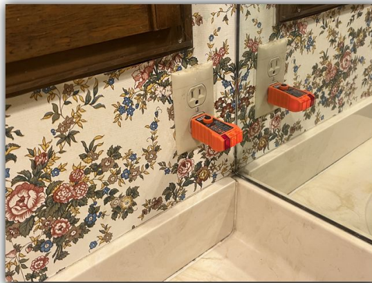
Missing GFCI protection in bathrooms
