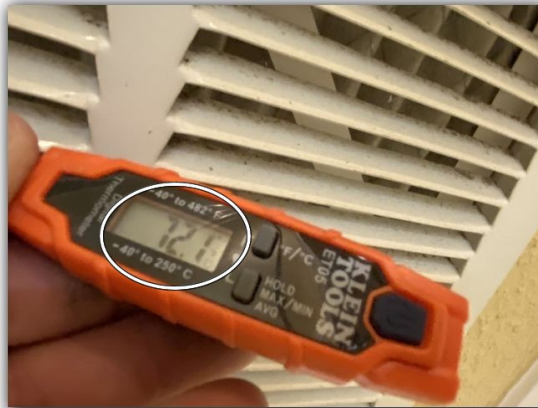
Return / room air temperature
