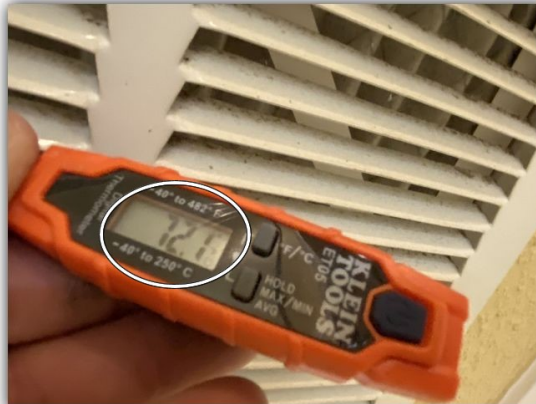
Return / room air temperature
