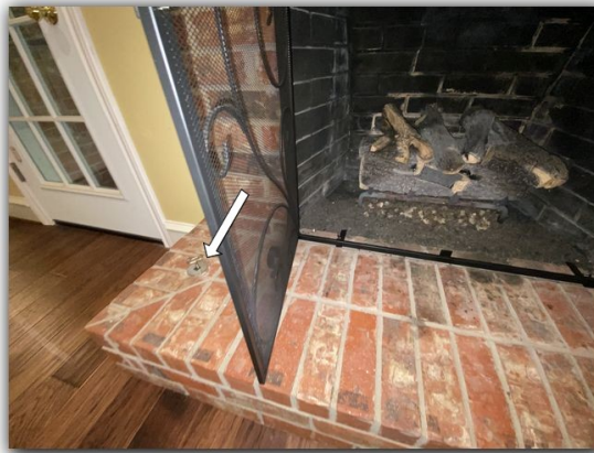
Gas working as should.
