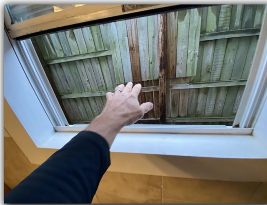
Various screens missing on home at time of inspection.
