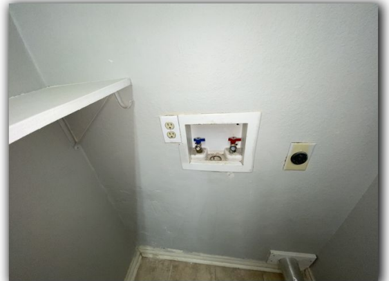
Washing machine drain
