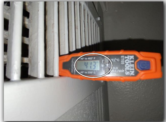
Supply air / differential
