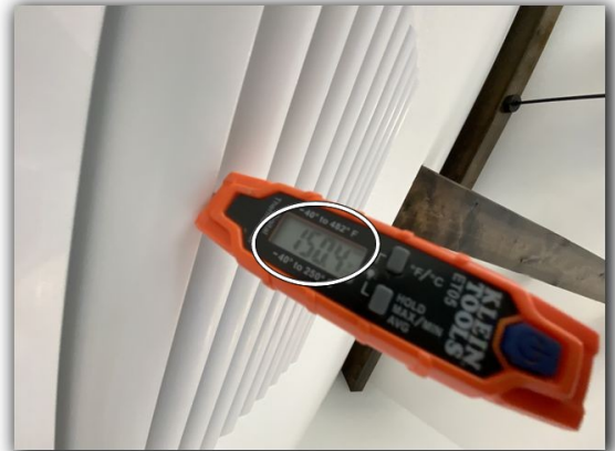
Supply air / differential
