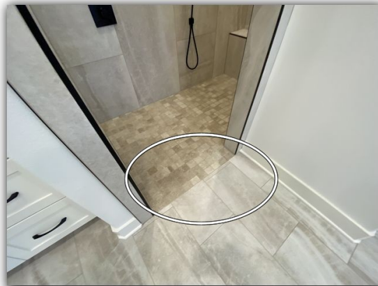
Ada compliant curbless entry
