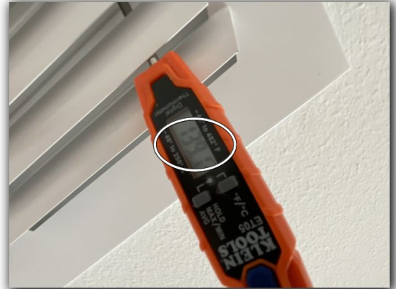
Supply air / differential
