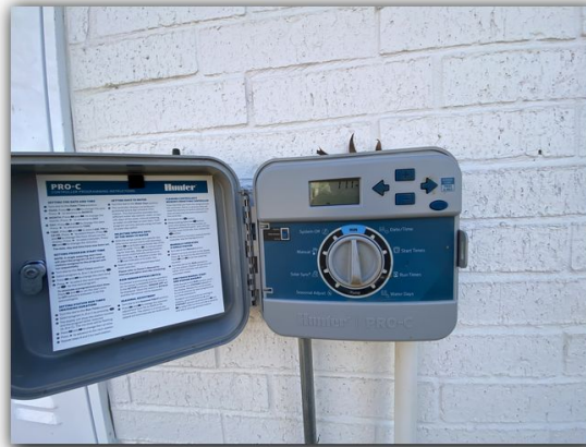
Hunter Irrigation system
